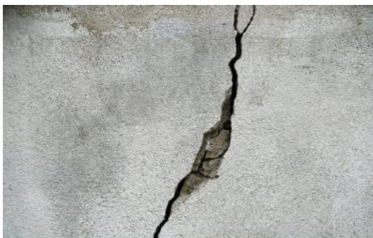
Figure 1: Crack in Concrete Element
