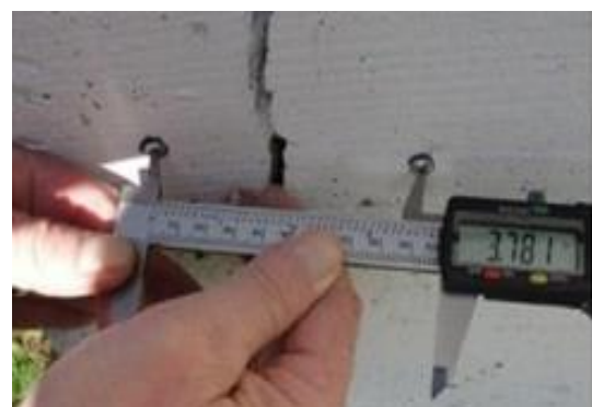
Figure 9: Measuring crack width using caliper
