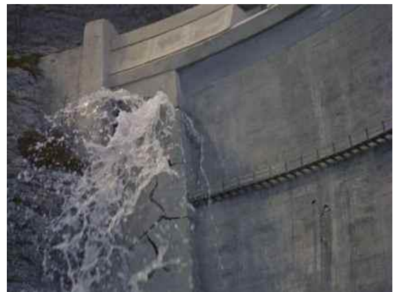
Figure 2: Crack in concrete dam
