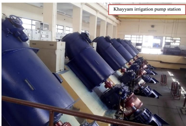
Fig. (10) Photograph of Khayyam irrigation pump station
