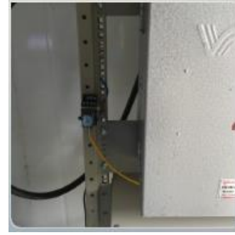
Fig. 5: Image of installing the warning device for running generator in case the generator is located inside BTS
