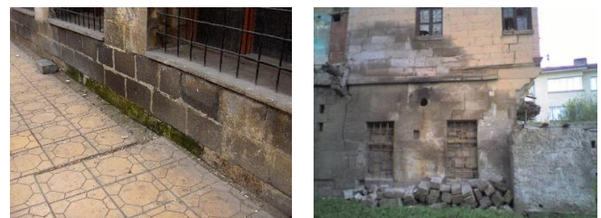
Figure 4. Wet areas on stone surfaces: color change, crusting, salt accumulation
