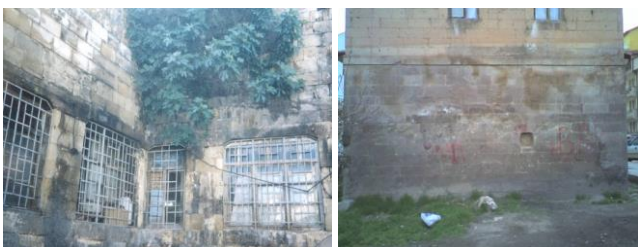
Figure 3. Examples of darkening due to air pollution in building stones
