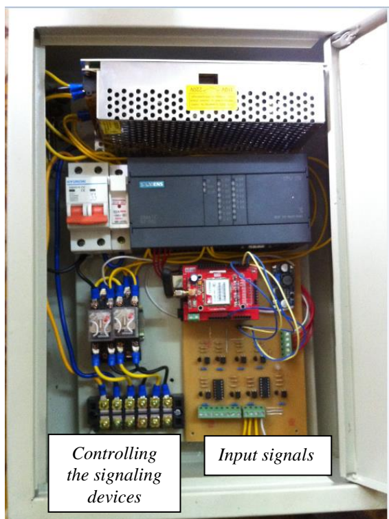
Fig. 11 Inside of control box
