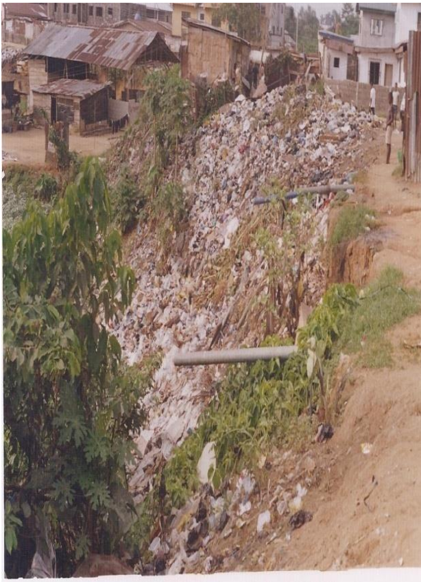
Plate 1: Municipal wastes dumped into the Borrow Pit (sewage pipes channeled directly into Borrow Pit)
