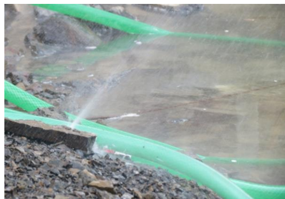
Leakage should be repaired immediately
