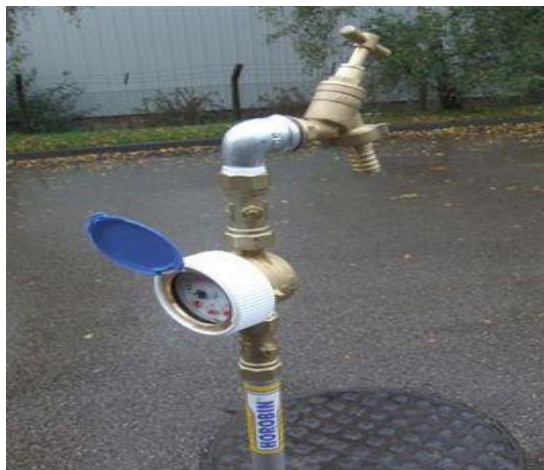
Water meter at construction site
