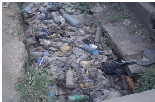
Fig. 8 Indiscriminate dumping of waste in drainage
